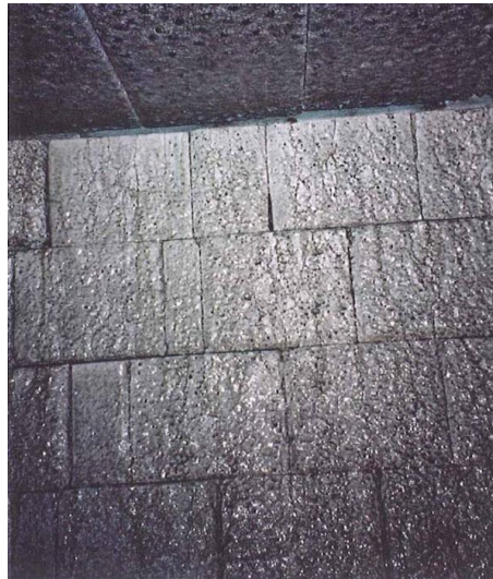
Superstructure corroded by volatile soda and phosphate
