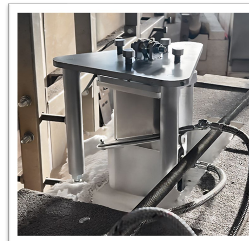
Installation on field
