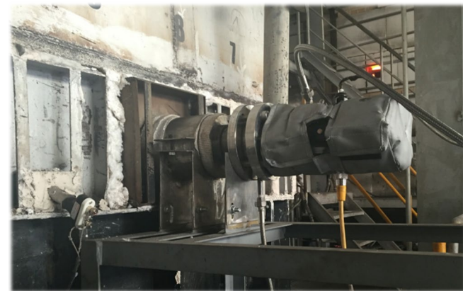
Stone detection camera installation
