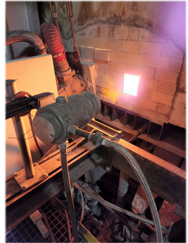
Water Cooled System
