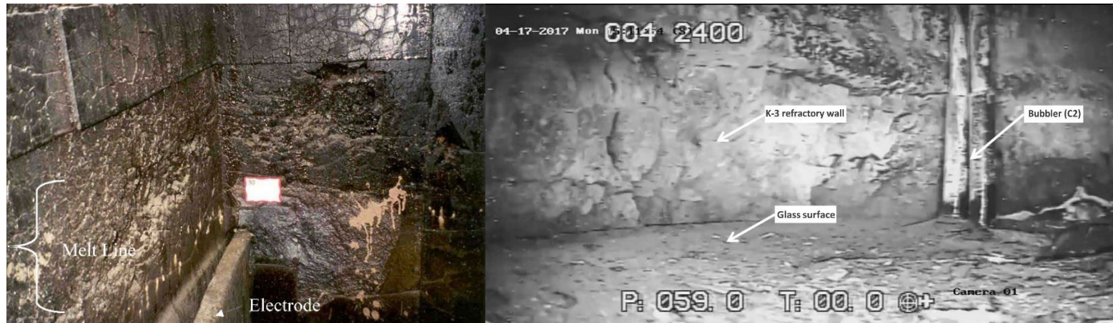
Corrosion damage of Monofrax® K-3 refractory lining of production melters: DWPF Melter 2 (left) [1], and SRS M-Area DM5000A (right) [2]
